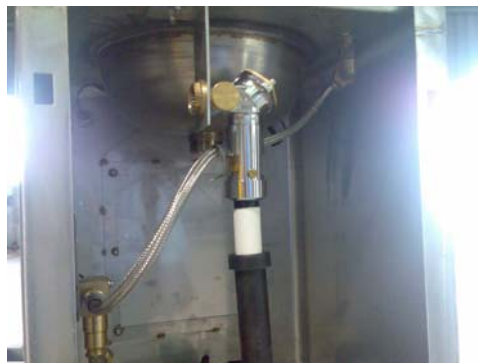
Typical installation in combi tower.
